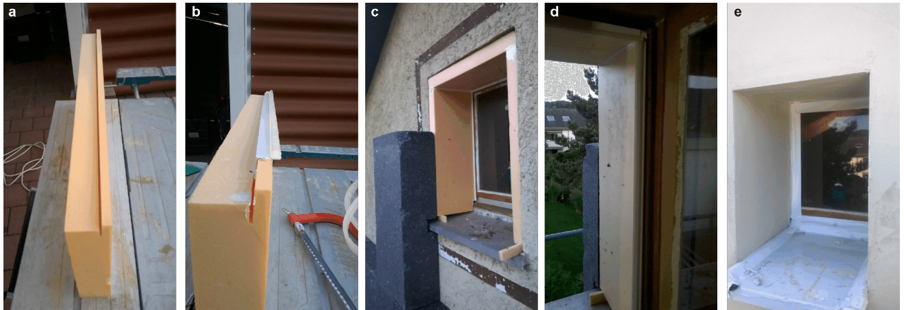
Figure 4: Insulation over casements: a) XPS board notched to size; b) PVC profile inserted with hose seal glued on; c) inserted in the reveal; d) interior view; e) exterior view after plastering
