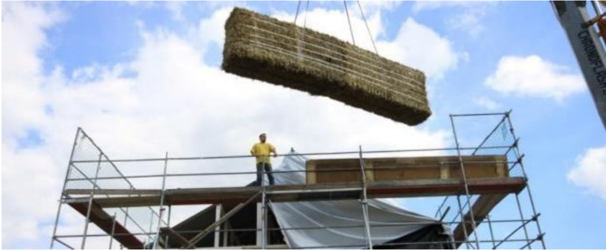
A crane had to be used to move the approximately 300 kilogram straw bale so that it could be used as insulation for Benjamin Krick's house. The straw bales came from the field next door.
